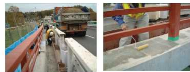
Fig. 1-4 Concrete barrier of bridge to which a silane surface impregnated material is applied
